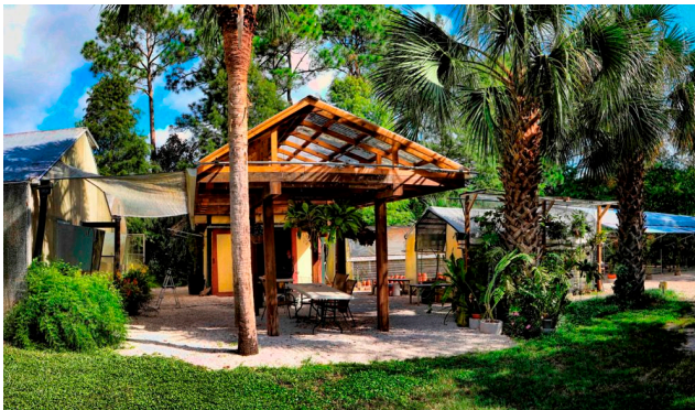
A potting shed and pergola added. Now, what are we going to build in that old vegetable garden?
