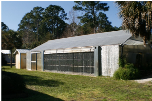
Retractable curtain added for air movement.
