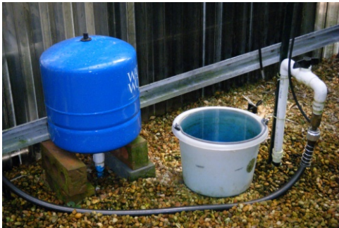
5. Pressure Tank and Siphonex System
