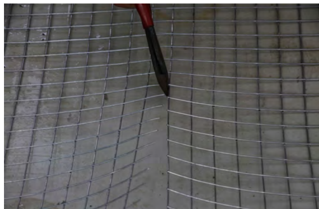
5. Snip away, use nippers to cut flush along the edge of the wire.
